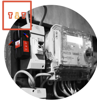
MCB/ DISTRIBUTION BOARDS
